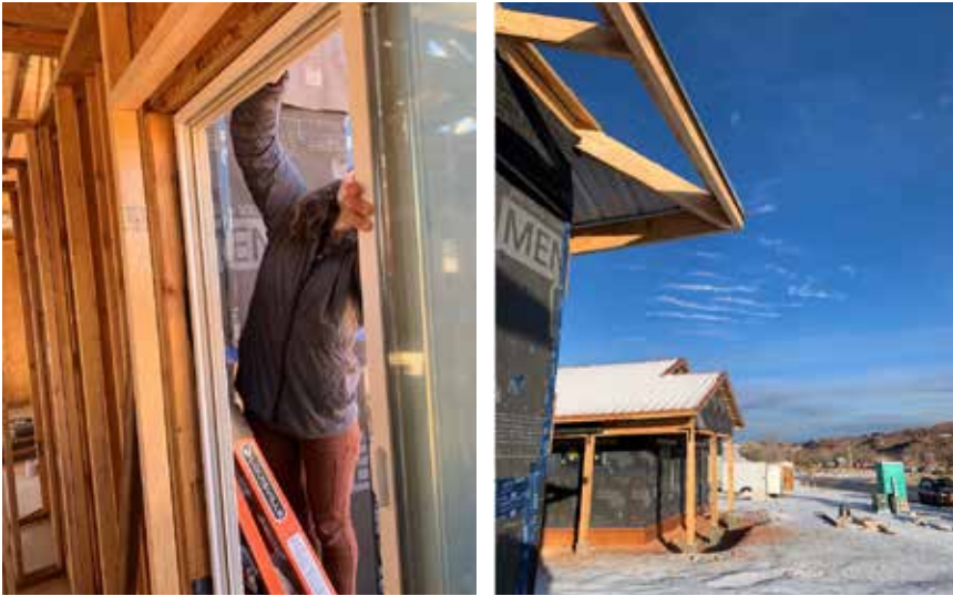
Figure 4. (Left) Picture displaying double studding method of construction, Community Rebuilds (Right) Two Community Rebuilds homes after being house wrapped.
