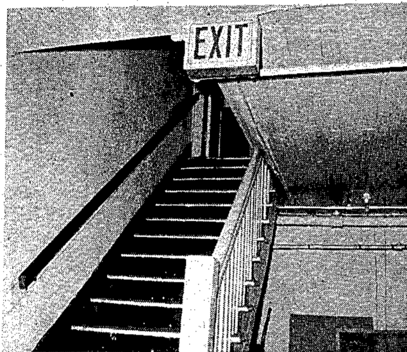
The cracking stairway entrance to the lounge area is in need of lighting and color. Repeated attempts to advertise the lounge by signs have been frustrated.
